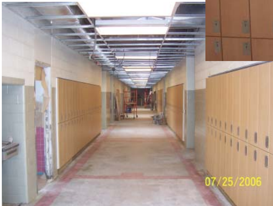
New lockers and lights are installed for a fresh and bright look
