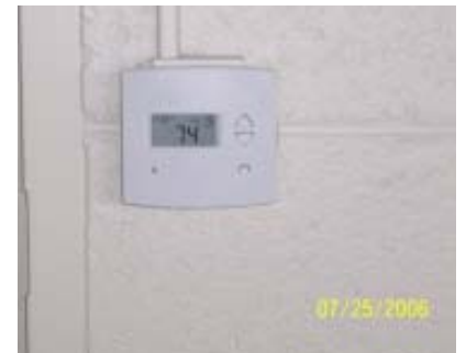
A new thermostat is installed in the library and each classroom and office to control the heat and new air conditioning
