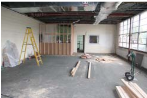
New Nurse's Office frame-in (left) access from the hallway - new small conference room with observation window (right) (This view is from inside the library)
